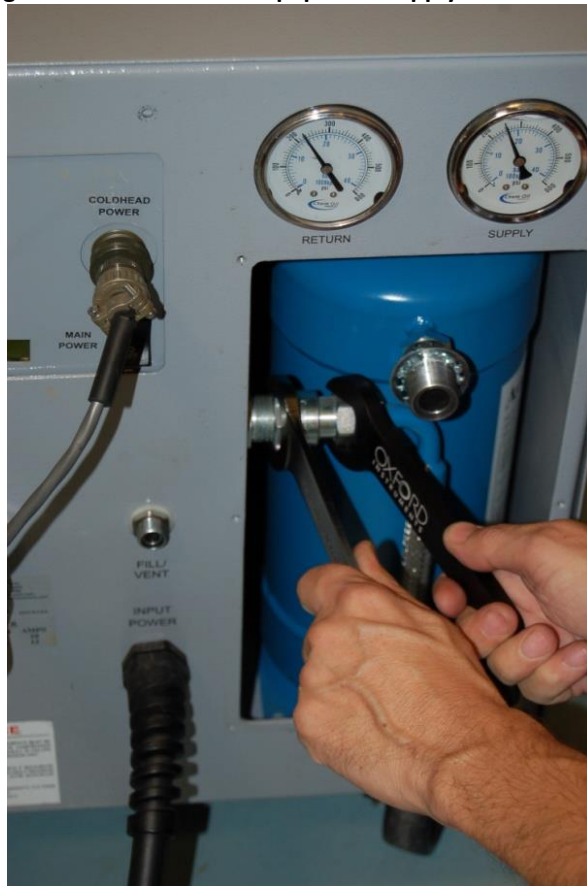
Figure 16 - Adsorber Aeroquip OMS Supply Line Removal
