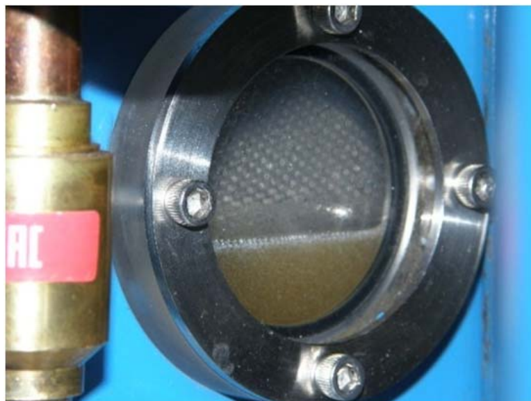
Figure 7 – Typical Sight Glass Oil Behavior During Operation
