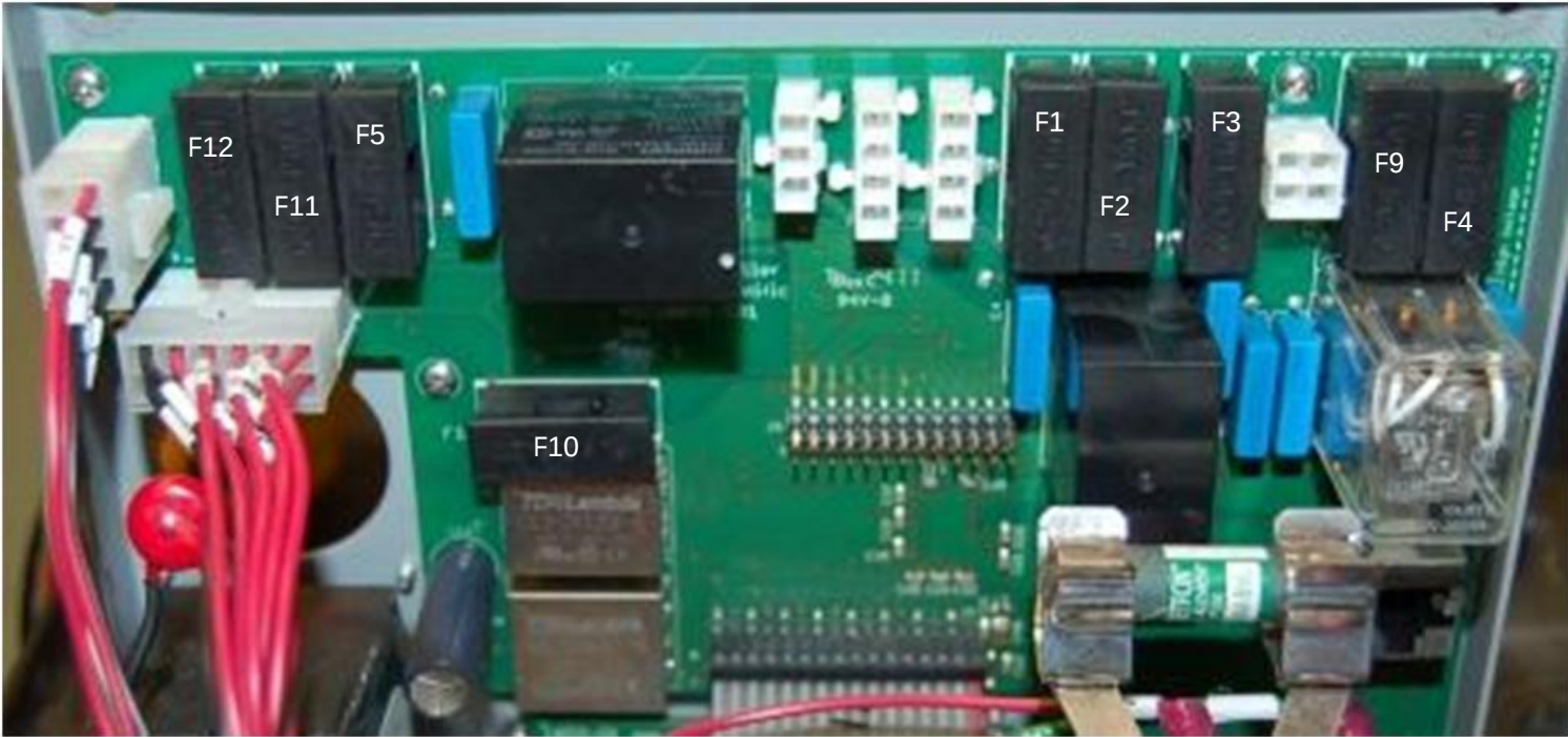
Figure 22 – M700RT Electronics Box Fuse Locations
